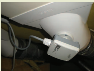
Ventilation double flux
